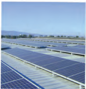
300-kilowatt Solar Power System
